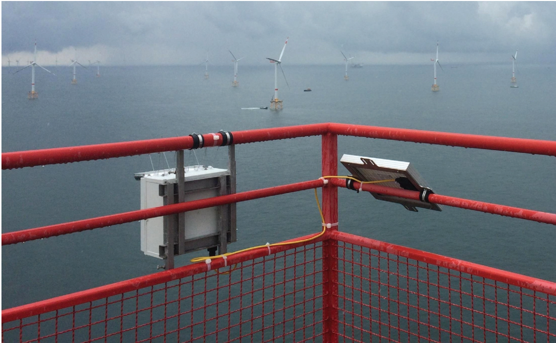
FIG. 2. Batcorder installed on the helicopter winching platform at the back of the nacelle of turbine II at approximately 93 m above MSL
